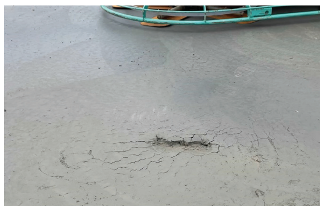
Fig. 2: Surface tearing during troweling
